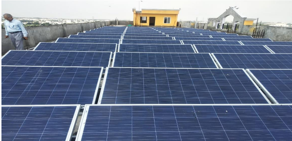
Figure 13 : Solar panels installed on roof
